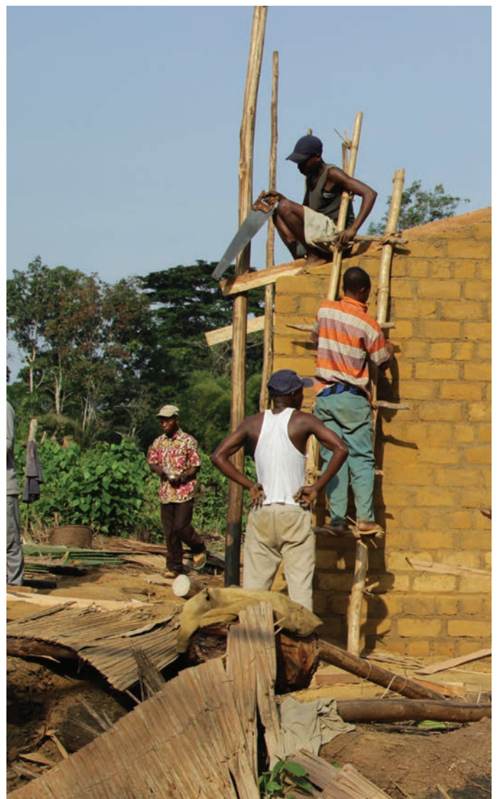
The building will feature brick walls that go up two thirds of the way to the ceiling to allow for unrestricted airflow in this tropical climate.
