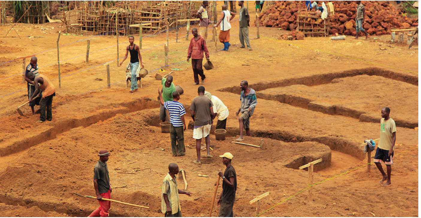
Workers are gaining new construction knowledge, which has the dual benefit of increasing sustainable livelihood opportunities for them and ensuring their ability to maintain the building structures, rather than outside contractors trekking to this remote area.
